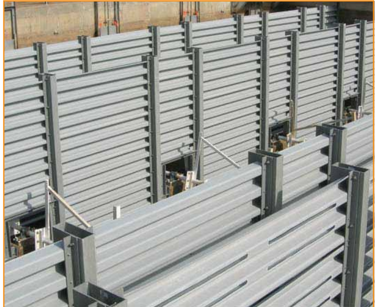
"D" structural baffle wall system - solid and slotted with FRP columns Sedimentation and Flocculation Basins
